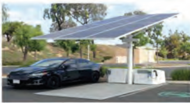
Solar Roof Panels
