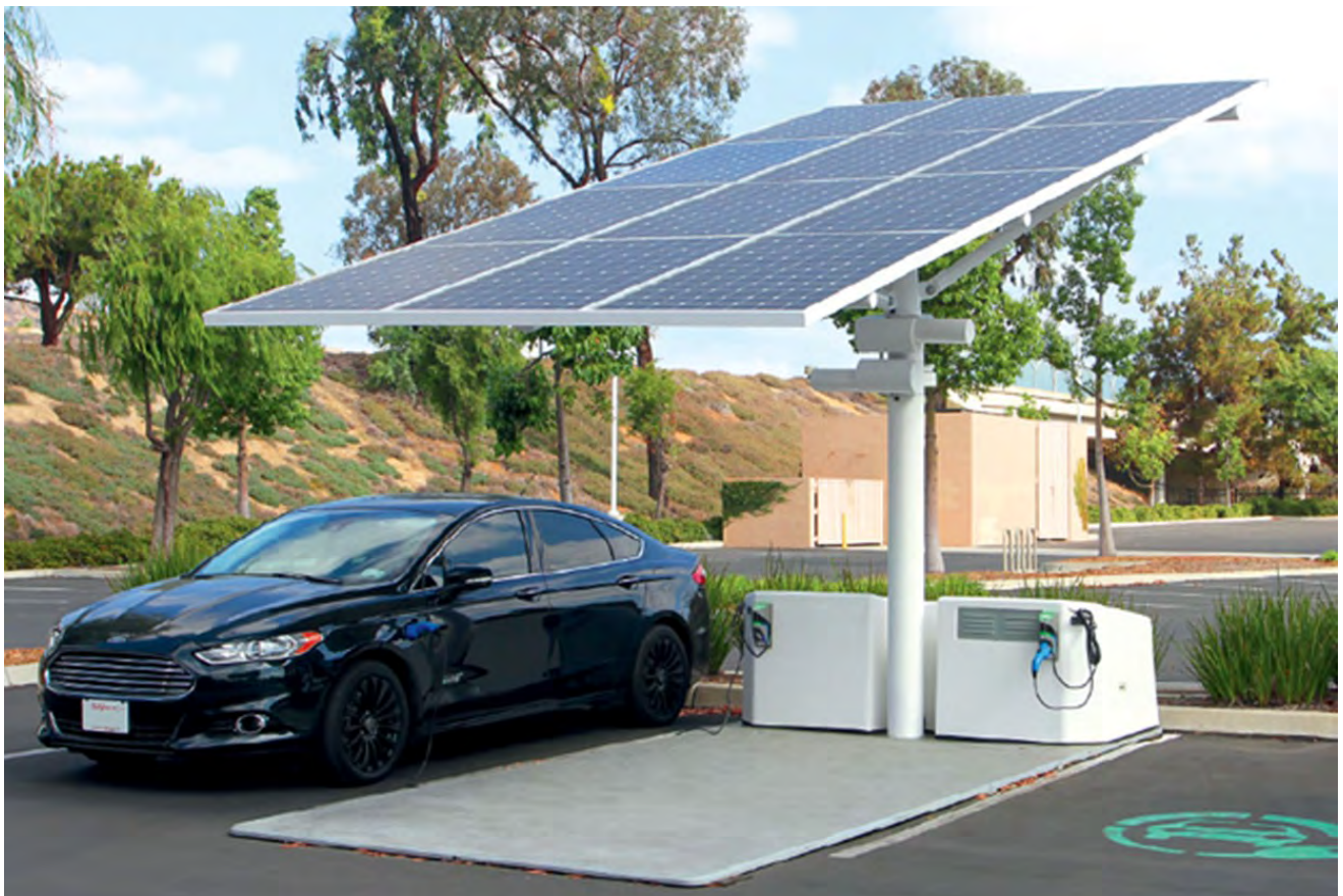
Solar-Powered EV Charger
